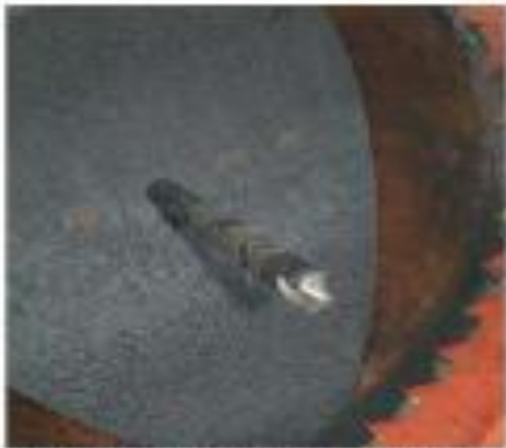
36" hot tap cutter, casing and pilot drill
